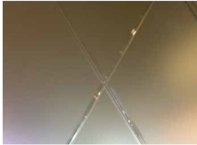
Custom Laminated Glass Panels: Installed with diamond pattern V-grooving for enhanced visual appeal.
