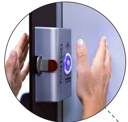
Sensor on interior of cubicle with safety release latch
